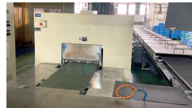
3D thermoforming facility / serial heating machine
