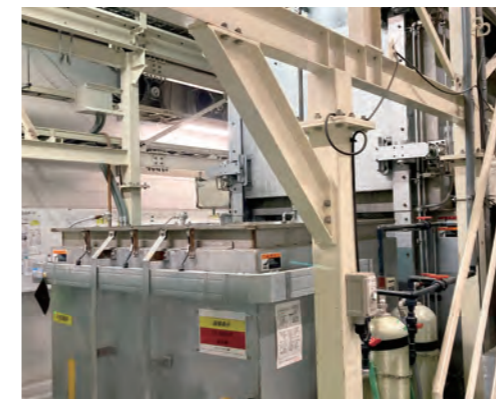
Tank to chemically strengthen
